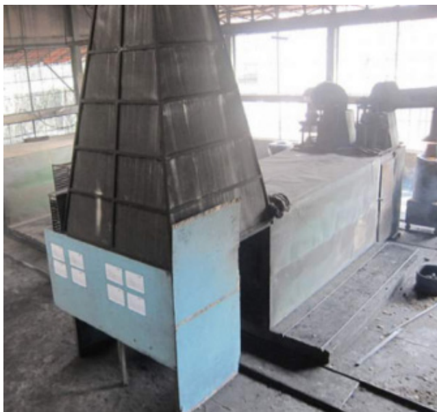
SGFE Tunnel Dryer. Photo: Carlo Figà Talamanca, SGFE.
